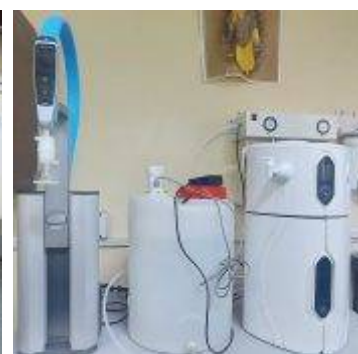
Water Purification System
